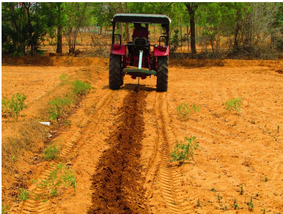
Well Recharge Pit
