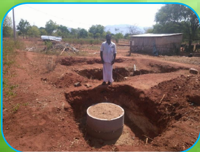
Well Recharge Pit
